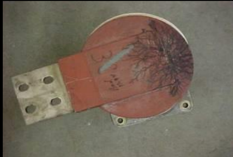
Manifestation of partial discharge on the switch
